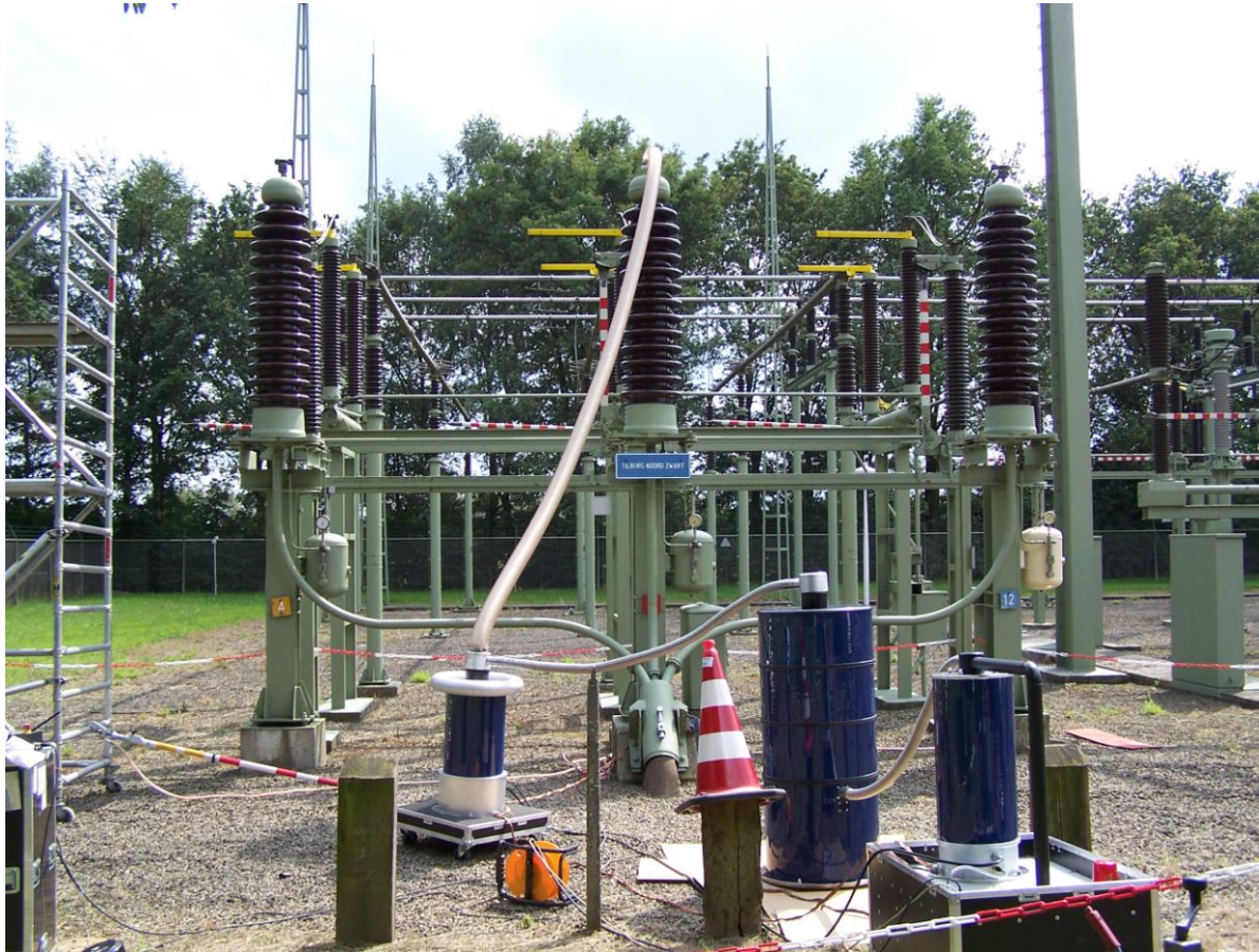
Testing 110kV external gas- pressure cable circuit ( 2.2 \mu\text{F} ), length 8.5 km using damped AC voltages (40 Hz)
