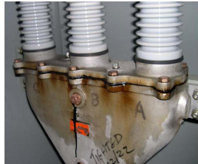
Figure A17: Vault 7U - Oil leak at gasket
