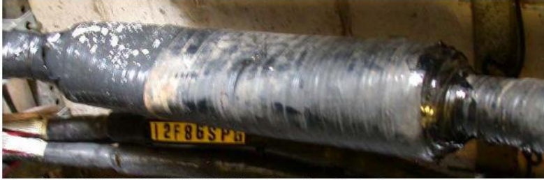
Figure B11: MH 363. Circuit 12F89. Splice collapsed and leaked.
