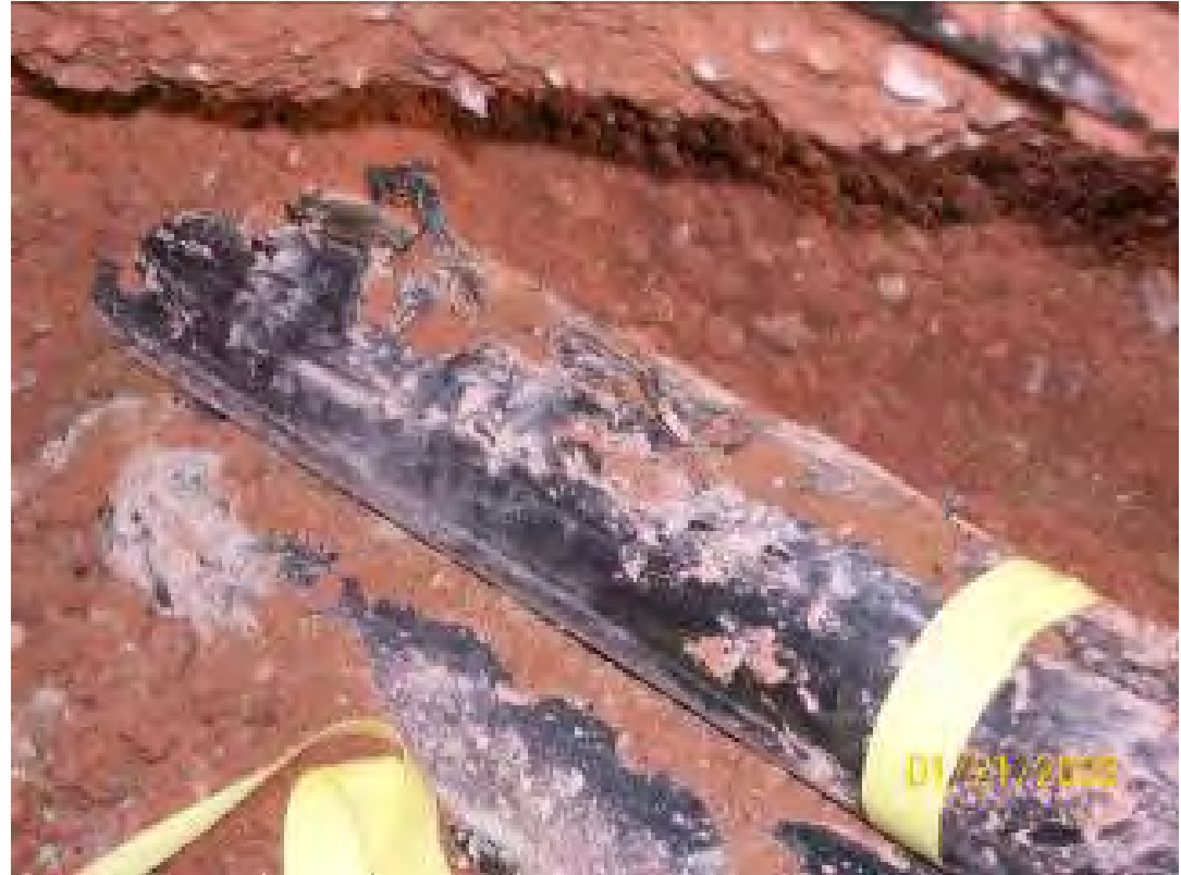
Cable defect was located within 3 inches on a 2000' cable.
