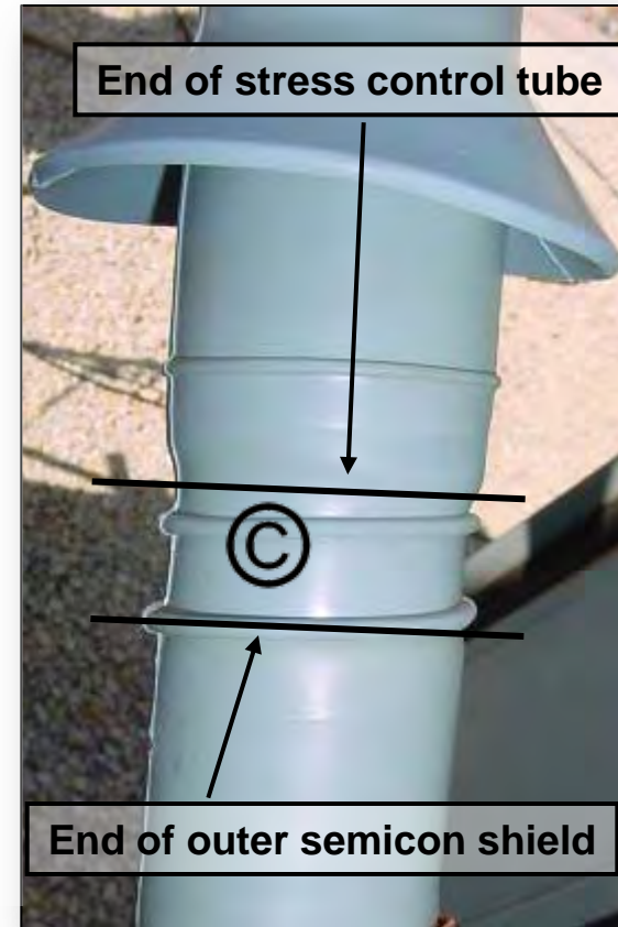
Example of misplaced stress material
