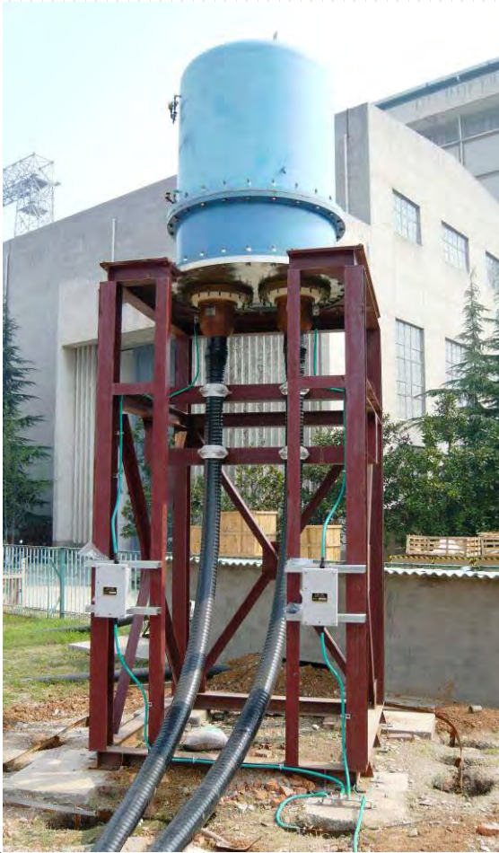
SF6 Sealing Ends
