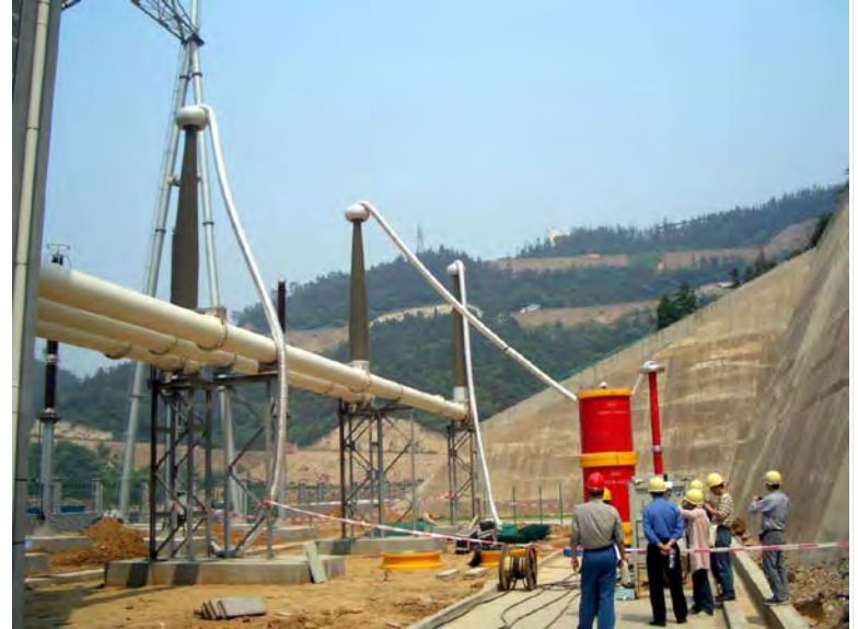
Testing view at 510kV AC for 1 hour.
